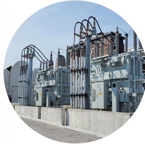
Perform inspections on critical assets
