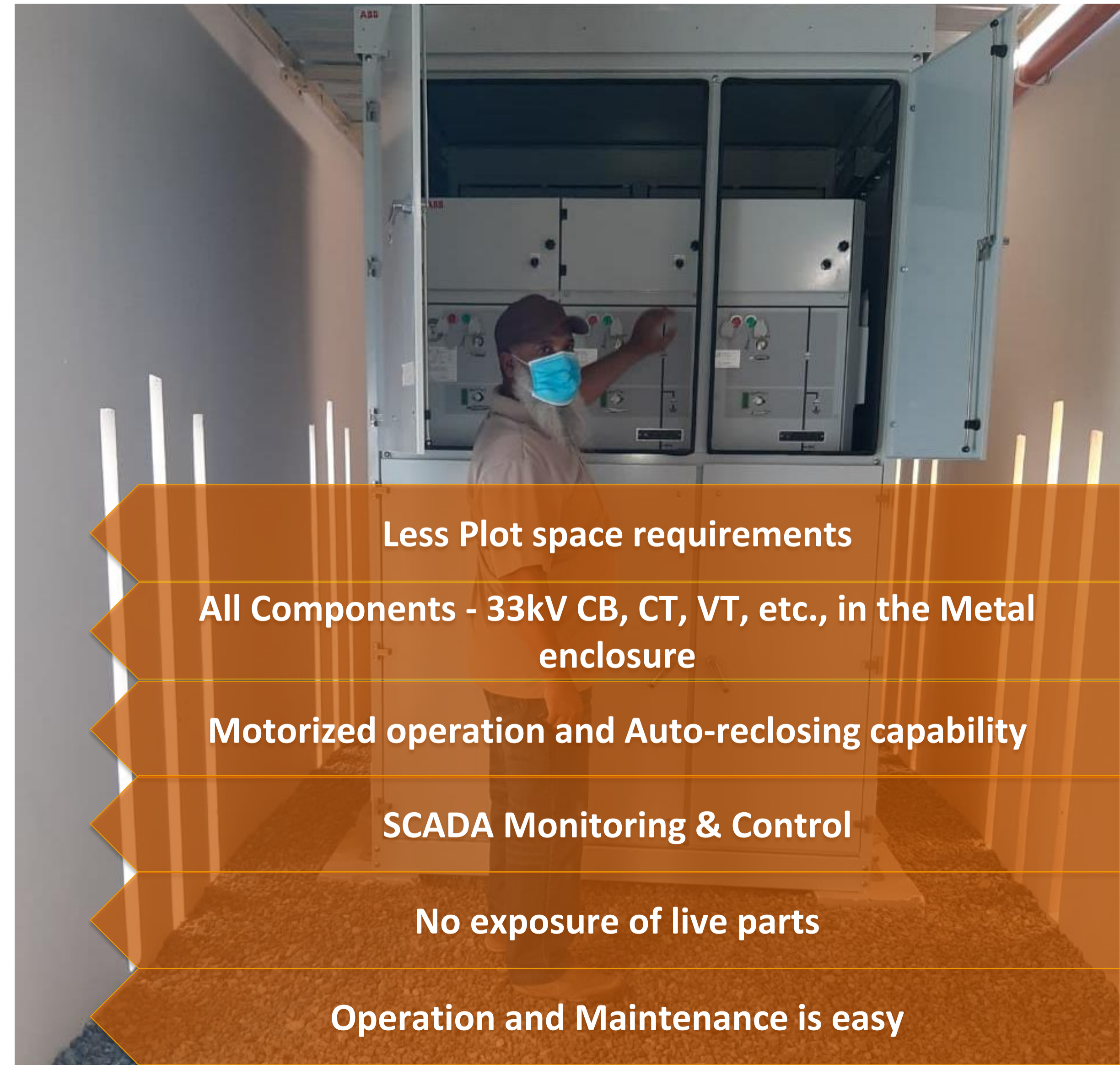
New - 33kV RMU Arrangements
